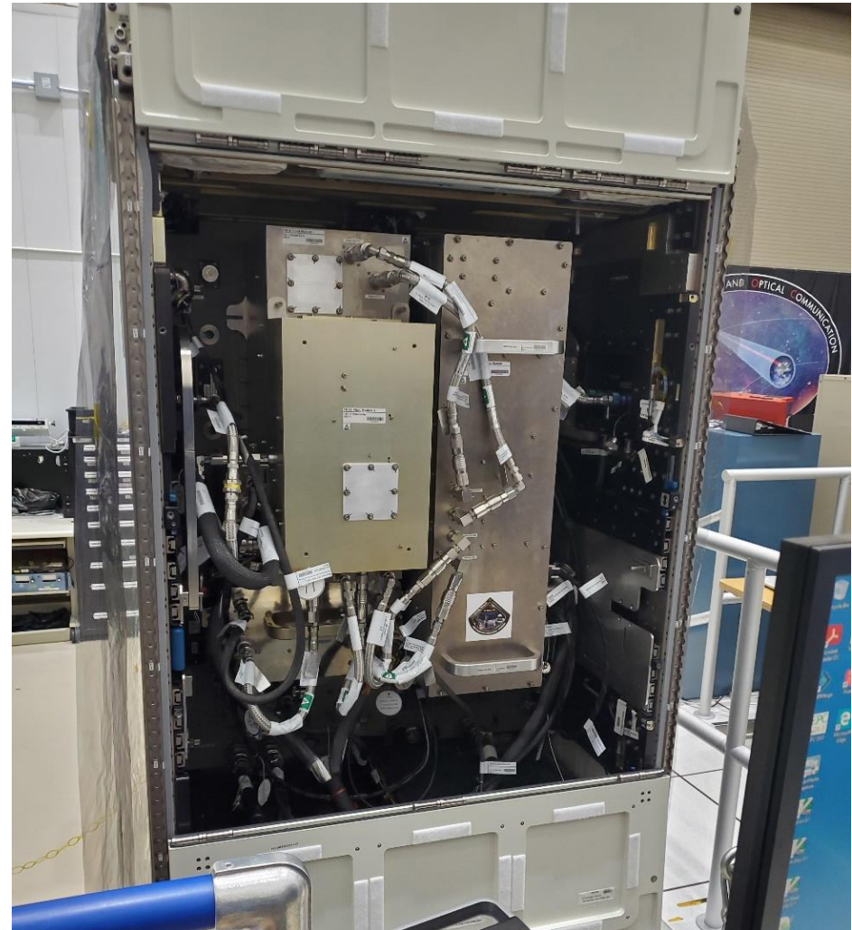
FBCE in the FIR Ground Integration Unit (GIU) at GRC
